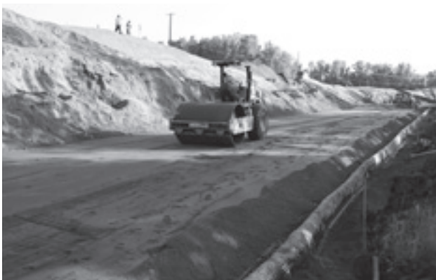
Heavy compaction equipment should be kept at least 3 ft from the face of the slope.
