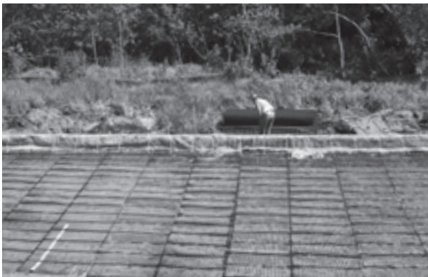
Installing the first layer of UX Geogrid perpendicular to the slope face.
