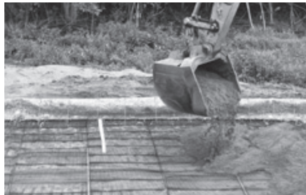
Fill should be placed and spread away from or parallel to the slope face.
