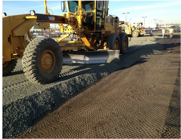
By installing TriAx Geogrid, approximately 15,000 cubic yards of aggregate base material was saved while also increasing the speed of construction.
