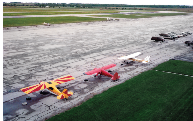
Severe cracking of the airport apron in 1992 at the Centralia Airport was likely to affect aircraft movement and safety.
