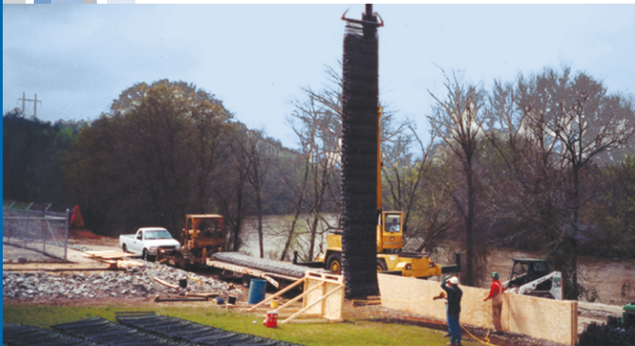
A 30 ft. Triton Mattress is lifted to place along the river's edge.
