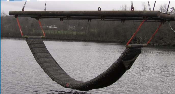
The Triton® System provided a sound foundation to support heavy piping.
